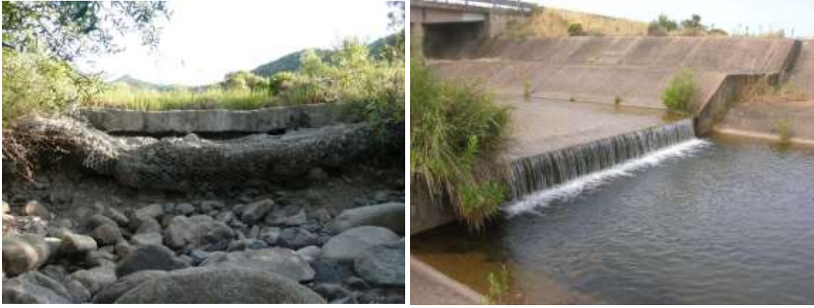
Figure 4. Dikes on Rio de Su Casteddu Stream: upstream (left) and downstream (right) Medau Zirimilis Lake.
